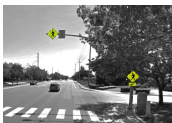
LED School Crossing Sign System – overhead mast & curb mounted
